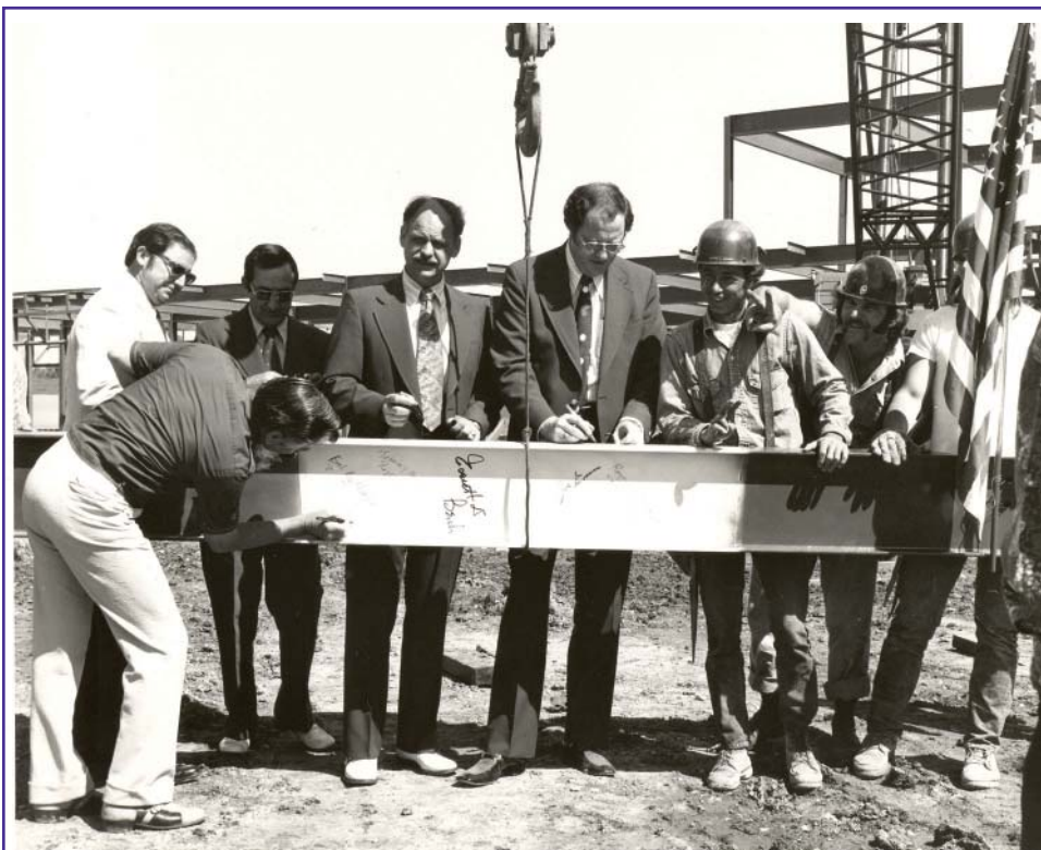
On April 17, 1974, the last beam was placed in the Veterinary Medicine Building. Painted red, white and blue, the beam was signed by (from left to right) Tom Beyt, project architect (standing at left in white coat); Joe Gossen, director, State Board and Building Commission; Dr. Everett D. Besch, dean; David Broussard, project manager and vice president, Eaton Construction Co.; and three steel workers. The person signing the beam is not identified.
